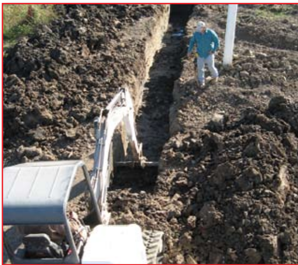
Trenches are dug to supply power to the St. John Outpatient Clinic site.
