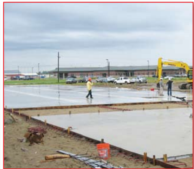
Concrete cures as the plotting of the module-aided site begins to take shape.
